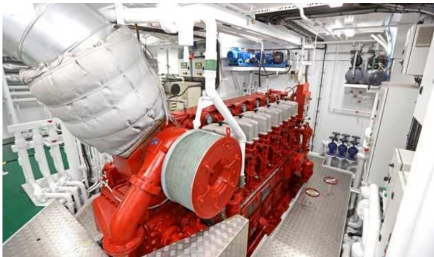
▲ General view of Alannah Riley's aft engine room.
