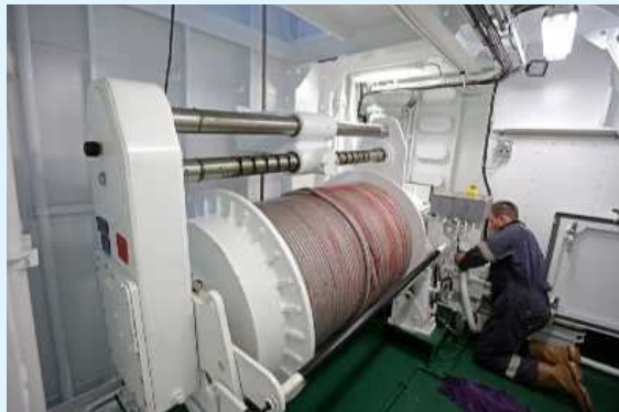
Rapp Marine engineer Drew Elphinstone commissioning the aft starboard split trawl winch.
